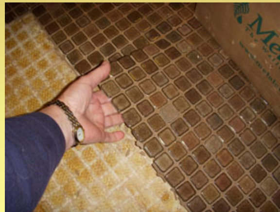
Small tile leads to a lot of dirt collecting in the grout lines
